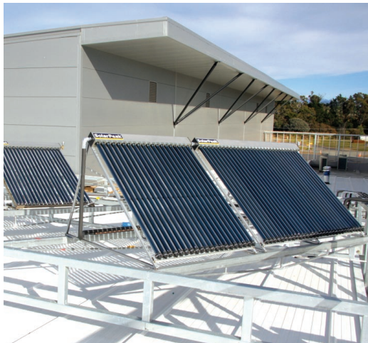
Vacume Tube Solar panels on Apollo’s Yealands Project
